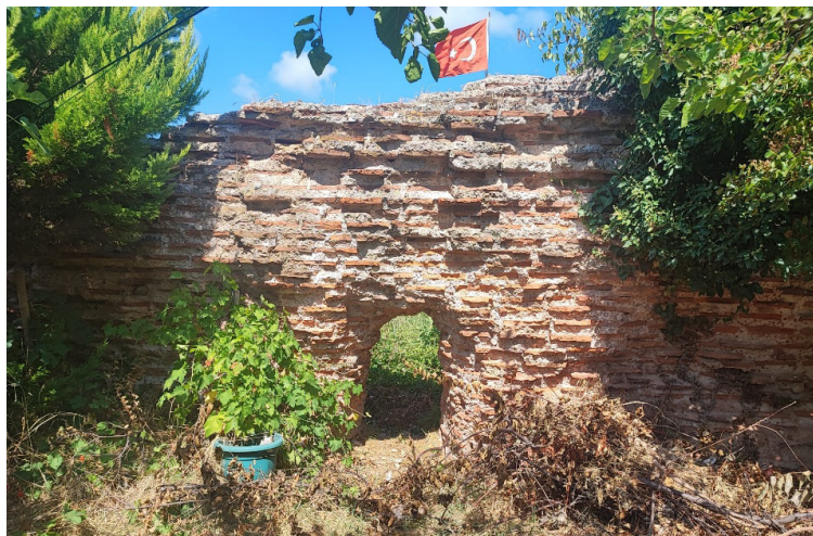
Figure 10: A section of the wall built using a technique with rows of bricks and rubble masses.
